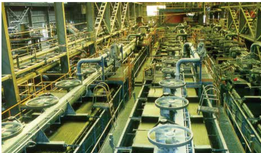
↑ Typical mine flotation plant
