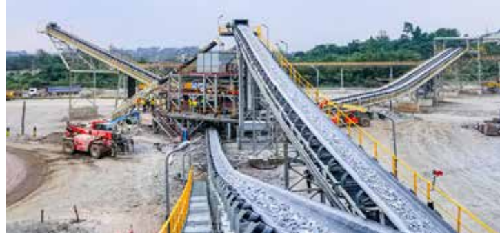
Carbonate Plant Expansion Project (Ghana) Client: Ghana Manganese Company Scope: Supply, Fabrication & Installation of 530m of Conveyor Gantries
