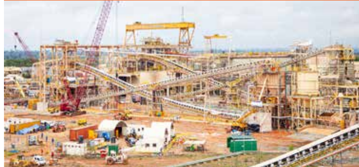
Scalable Ahafo Mine Expansion Project (Ghana) Client: Newmont Goldcorp Scope: SMPP Installation including Ball Mill Installation
