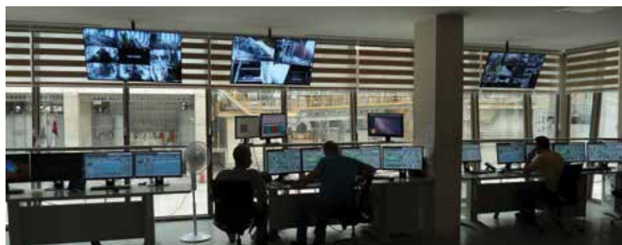
↑ Figure 6 - Central Control Room – Cement plant in Soma, Turkey
