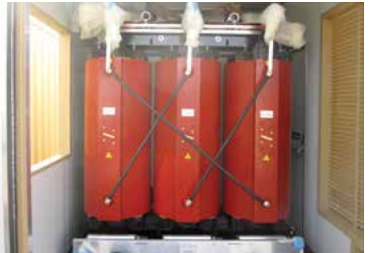
→ Internal view of a modular substation including a 2 000 kVA cast resin transformer
