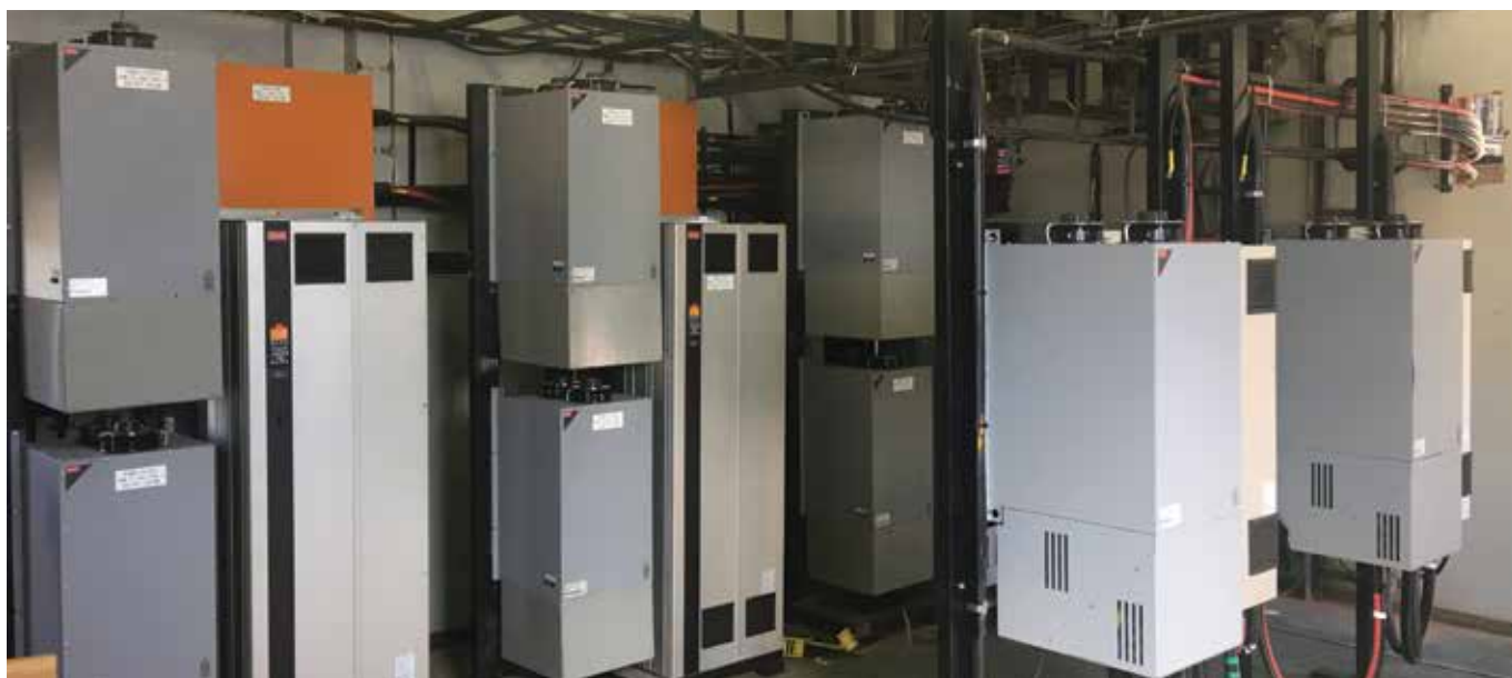
↑ The process cooling water (PCW) system has saved the company millions in operational costs
