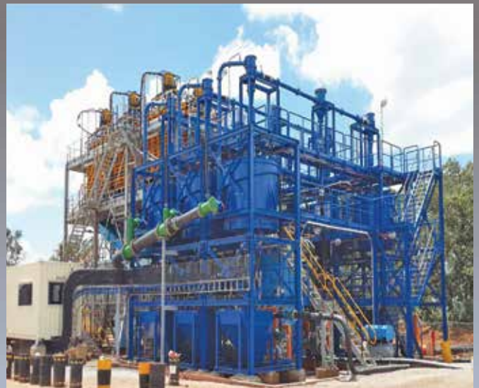
Copper Fines Recovery Plant
