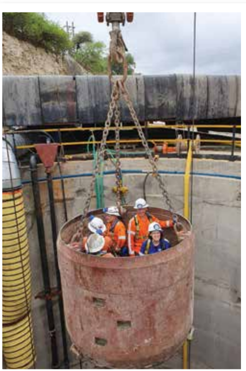
↑ Editor Laura Cornish travels by kibble with the Murray & Roberts Cementation and PMC team down the new ventilation shaft under construction late in 2019
