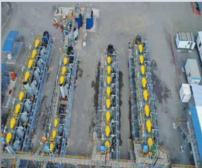
Lump sum Turnkey PGM Concentrators`
