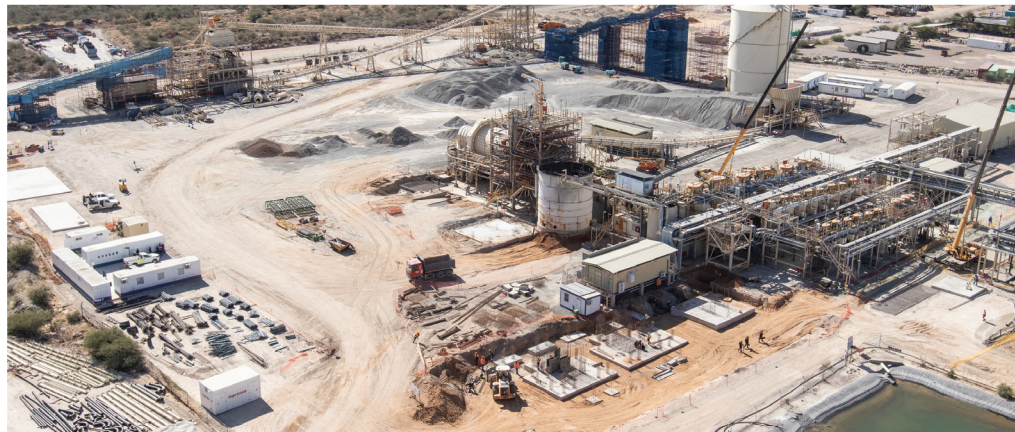
↑ The scope of Concor's work at the Boseto process plant includes earthworks and concrete civils to the existing plant and for the new process plant structures for the crushing, milling, flotation and concentrate handling circuits
